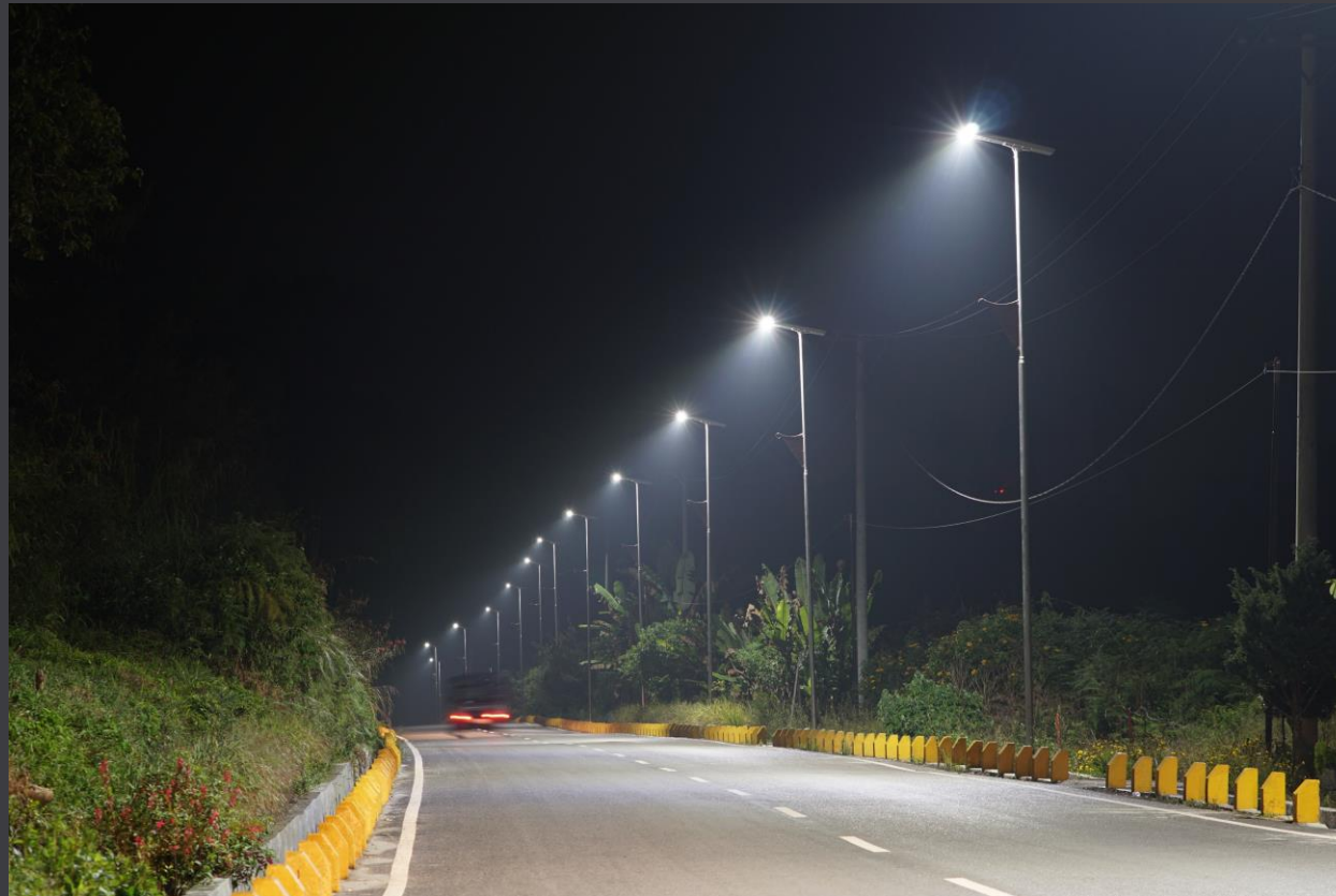
Solar lights address the challenge of public lighting in a dramatic landscape in North Sumatra, Indonesia
