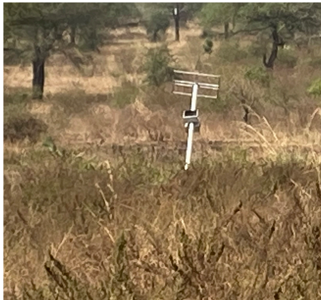
Vandalized Solar Light, Rhino Camp Settlement, Uganda, 2022
